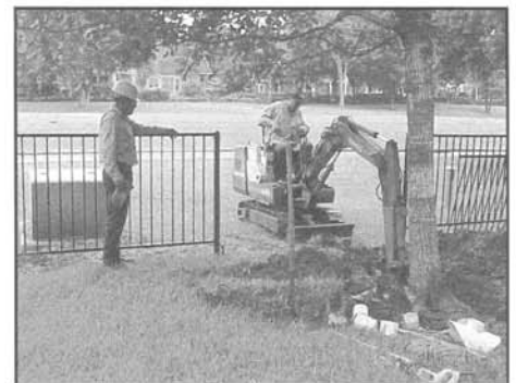
Paul Segura, Field Crew Leader (on tractor), and Jose Nunez checking sewer tap on the main line in easement.
